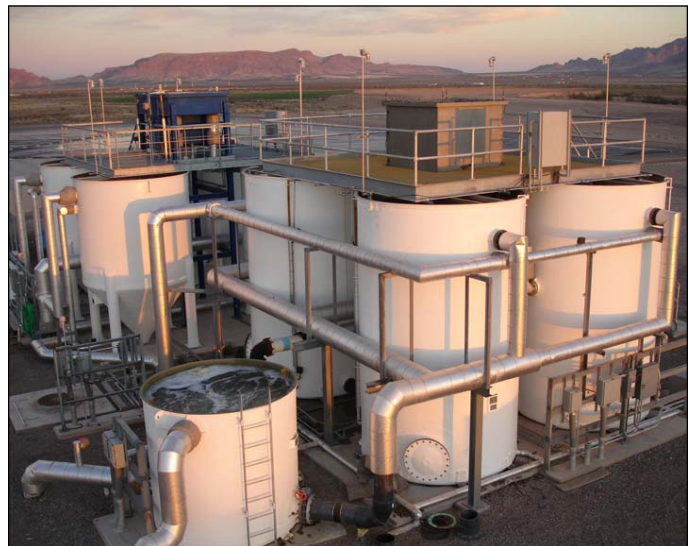
Water Reuse Installation
