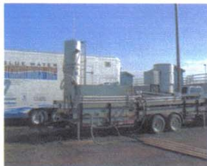
■ A mobile pilot trailer provides a water treatment system that can be relocated once the remediation project is completed.
